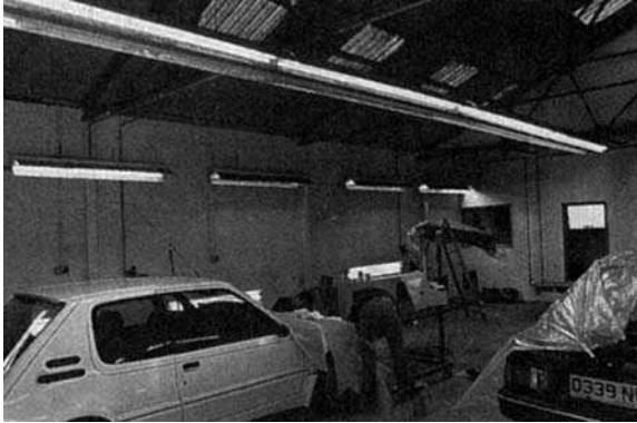
Figure 15.3 Lighting used in the stripping and straightening areas ( Fifth Generation Technology Ltd )
