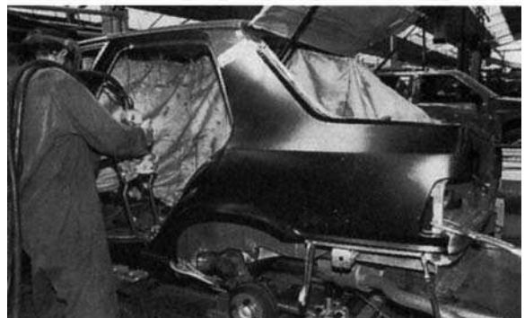
Figure 10.19 Pincer welding gun used in different locations in repair work ( Motor Insurance Repair Research Centre )
