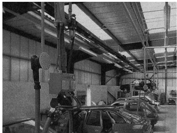
Figure 3.67 Dust extraction system in a workshop (Minden Industrial Ltd)
