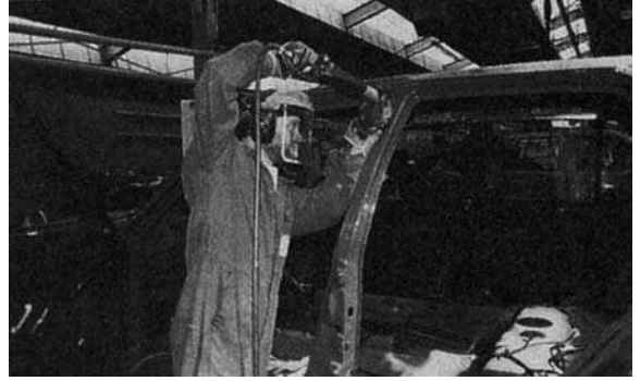
Figure 14.97 Cutting out damaged panels with a power saw ( Motor Insurance Repair Research Centre )
